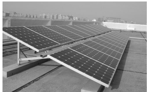
Fig.4. Operational PV power system on the rooftop of Building A of Hojing Elementary School.
