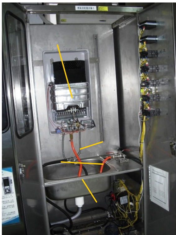
Figure 3. The internal configuration of the gas consumption measurement system entity
